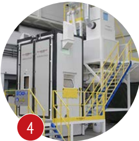
Closed-Loop Media Recovery Cyclone, dust filtration, and vibration sieves for clean and continuous recirculation.
